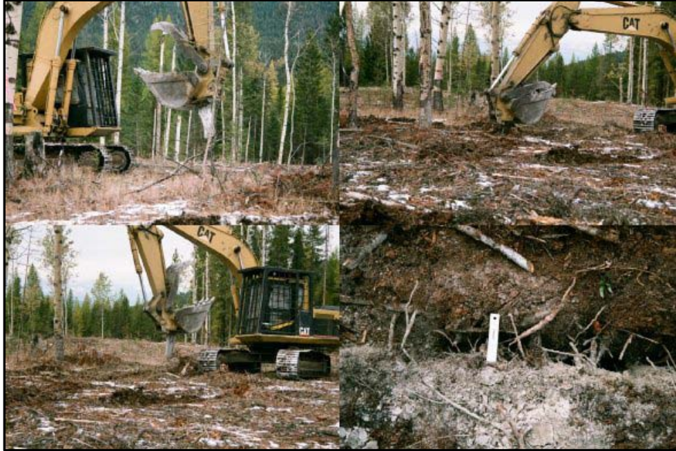
Figure 6. A montage of the root trenching process on the aspen firebreak unit. The upper left image is of the backhoe with the cutting blade attached to the bottom of the bucket. The upper right and lower left images are of the blade being pulled through the ground around the base of the aspen trees. The image in the lower right is of the resulting trench with the ruler indicating the width of the trench. A large number of severed roots are visible in the image.
